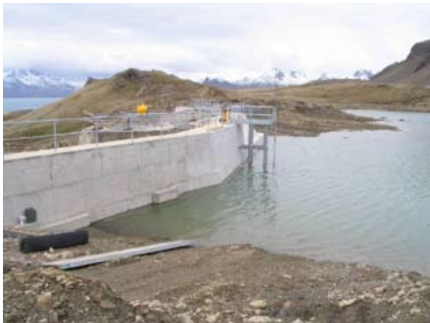
South Georgia hydroelectric scheme, 200kw output displacing 250m 3 of diesel a year - active since December 2008
